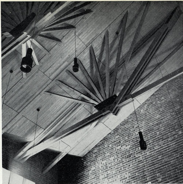
Detail of the roof construction in the council chamber in the Town Hall at Saynatsalo (1952)
